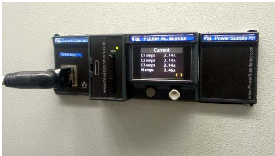
Photo 2 - Sample Caption - PQube installation at sample customer
